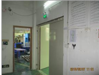
Photo of fire safety equipment Emergency exit.JPG
