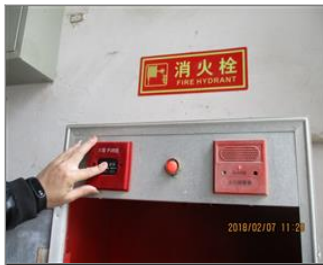
Photo of fire safety equipment Testing for fire alarm.JPG
