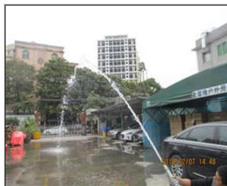
Photo of fire safety equipment Testing for fire hydrant.JPG
