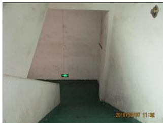
Photo of fire safety equipment Escape staircase.JPG
